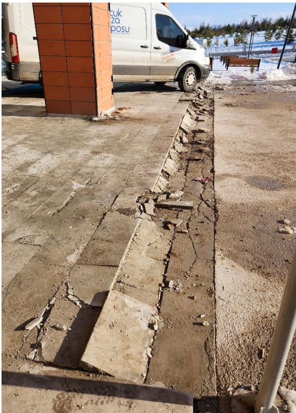
Damage to tilework at moat perimeter
