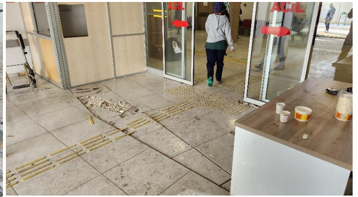
Damage to floor tile at emergency entrance
