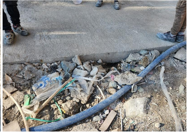
Construction debris restricting movement at moat cover perimeter
