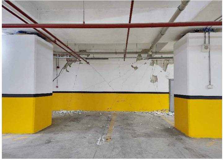
Basement wall damage due to lack of movement joint
