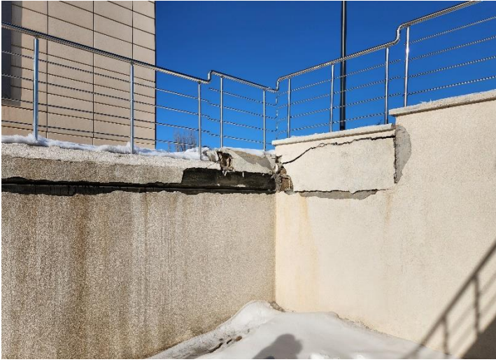
Damage due to no movement clearance between isolated structure and retaining wall
