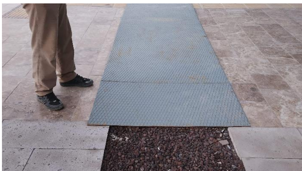
Movement joint at front entrance and crushed pumice stone used as moat infill
