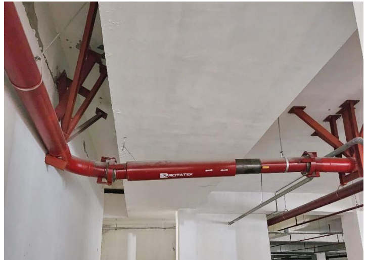
Damage to piping system support due to incorrect function of flexible joint
