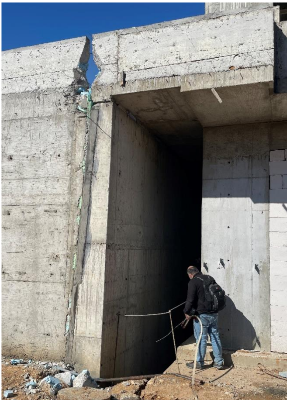
Damage at movement joint with inadequate clearance
