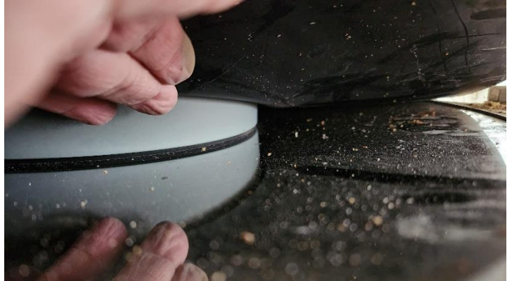
Close-up of isolation bearing slider unit below dust protection skirt
