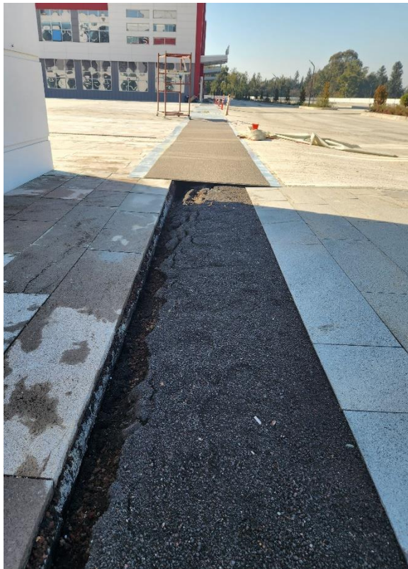
Moat filled with crushed pumice stone and signs of movement
