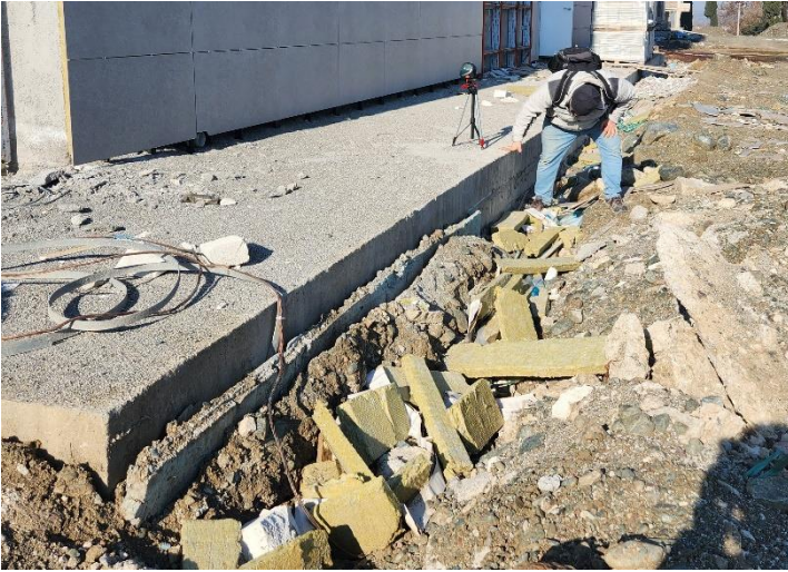
Construction debris and soil at perimeter joint
