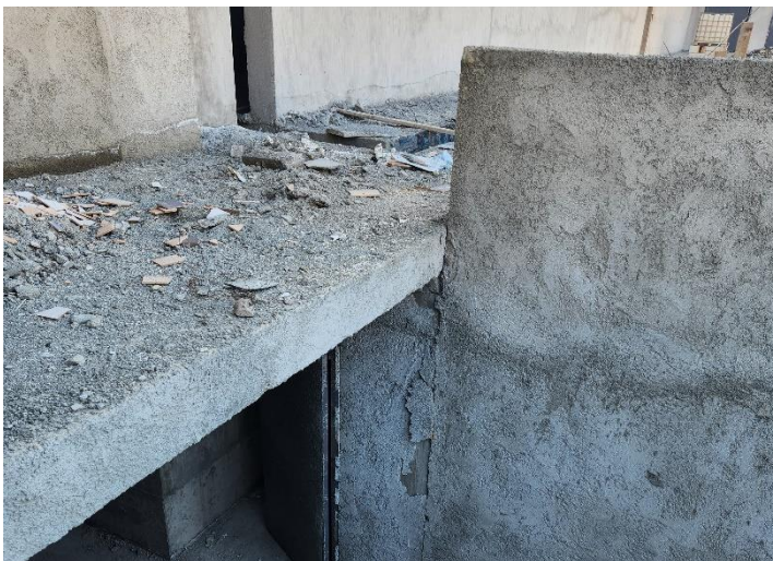
No movement clearance between perimeter moat cover and adjacent wall
