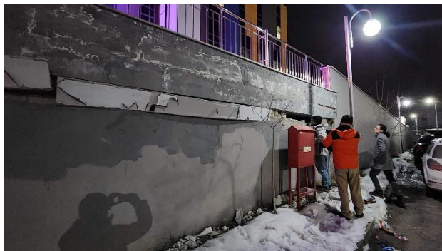
Damage at perimeter joint
