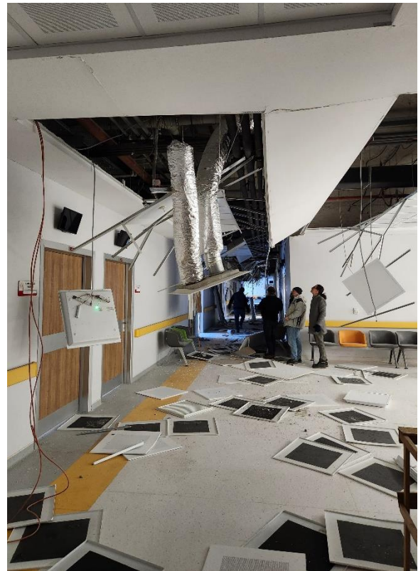
Suspended ceiling damage
