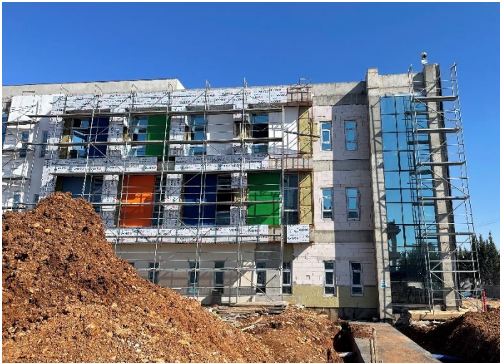
State of construction at time of earthquakes
