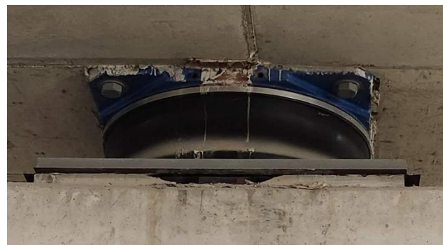
Grout cracking under isolator base plate
