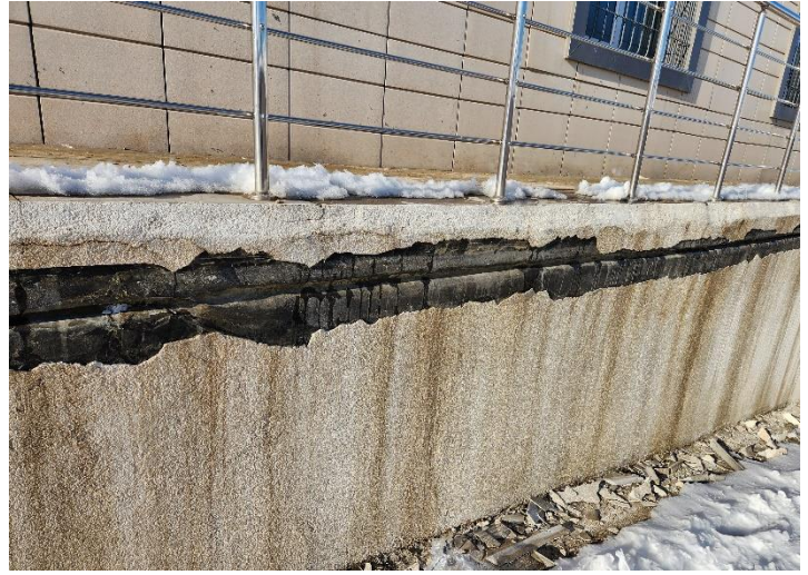
Spalling of plaster at perimeter joint
