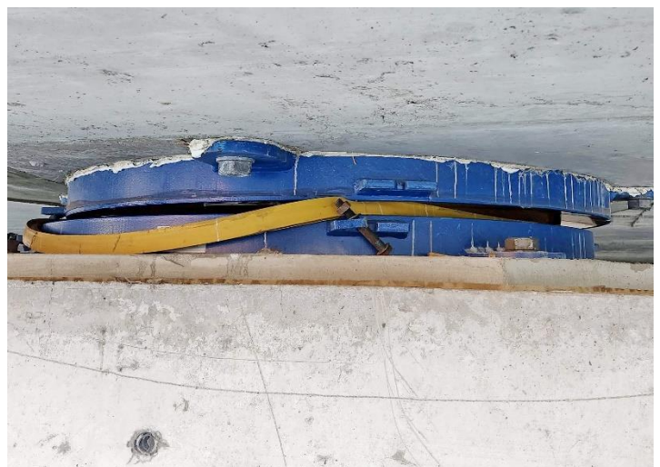
Isolation bearing with offset and disconnected shipping bolts
