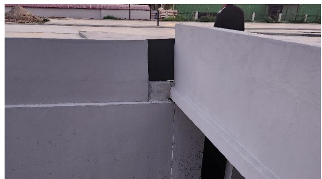
Inadequate movement clearance at pedestrian walkway
