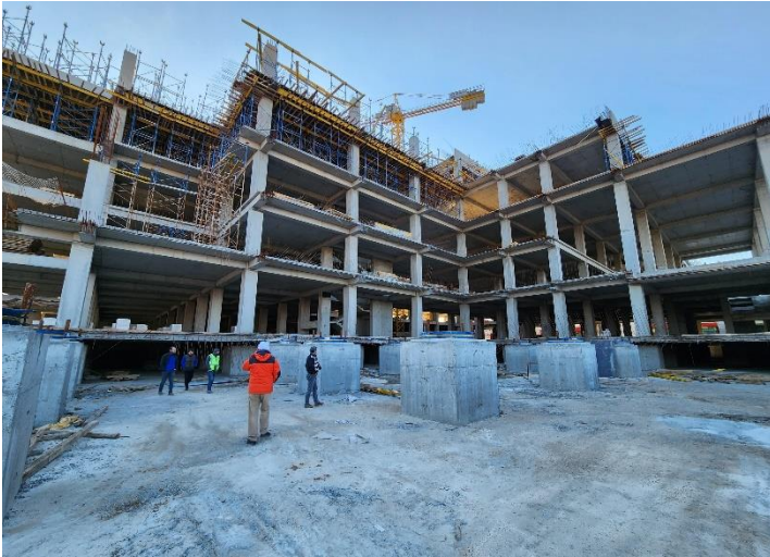
State of construction at time of earthquakes
