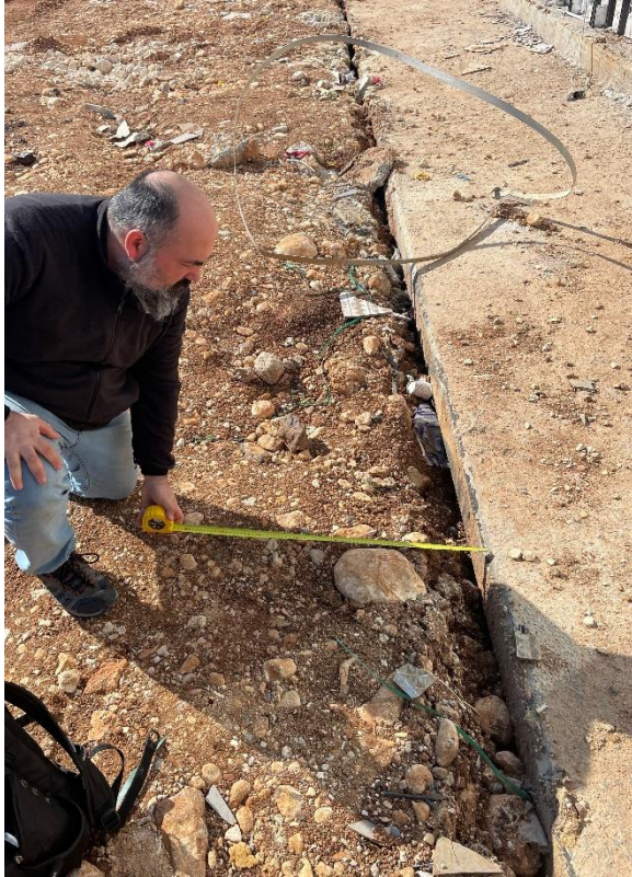
Soil movement at moat cover perimeter
