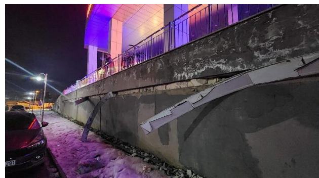
Damage at perimeter joint
