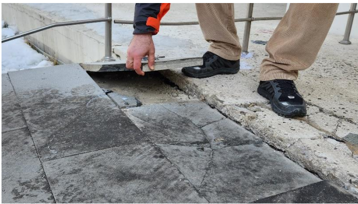
Damage to tile at entryway movement joint
